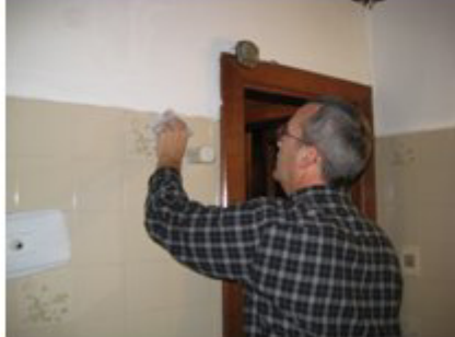
Steve and Stuart patched and painted all the bathrooms in the hotel, more than ten.
